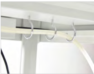
Neat hose arrangement
